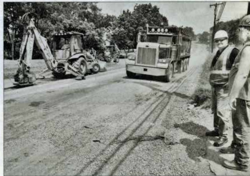
Daniel P. Creighton/The Mercury Mike McGourney, job superintendent, and Tim Sykes, foreman, with Danella Construction, inspect the progress of the water and sewer project on Farmington Avenue in Upper Pottsgrove. Work crews in the region will have it tough today as temperatures are expected to reach 100 degrees, with a heat index near 110.
